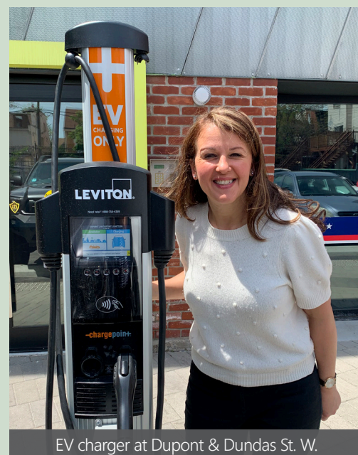
EV charger at Dupont & Dundas St. W.
